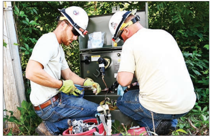
Above, Rock Energy workers access a padmount transformer at a residential home in one of the co-op's service areas.
