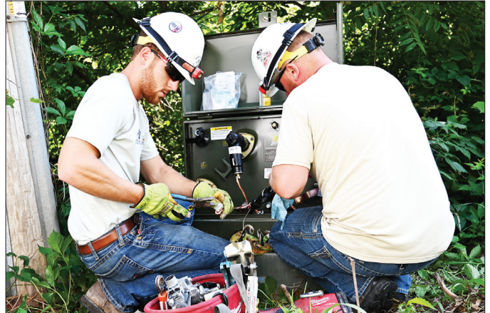
Above, Rock Energy workers access a padmount transformer at a residential home in one of the co-ops service areas.
