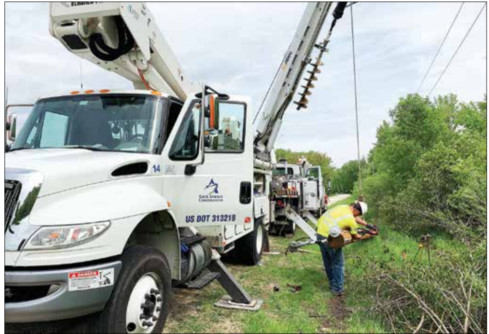
Rock Energy works diligently on line maintenance throughout the year. Pictured above, a Rock Energy crew works on a pole replacement project on Clover Road in Rockton, IL, in the spring of 2021.
