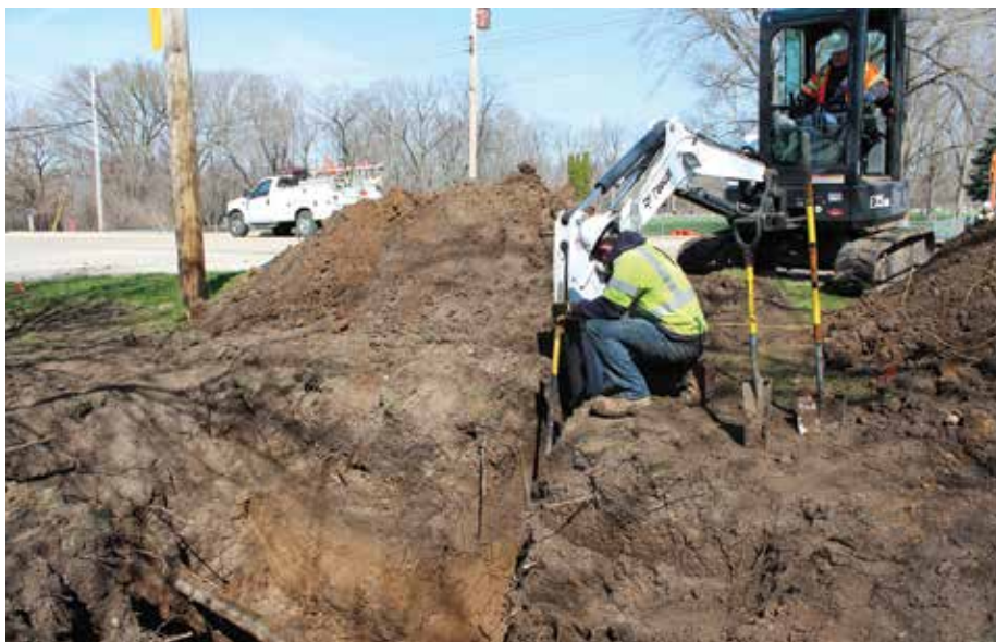
The natural gas crew replaces distribution pipe in Rockton to improve reliability and ensure safety.
