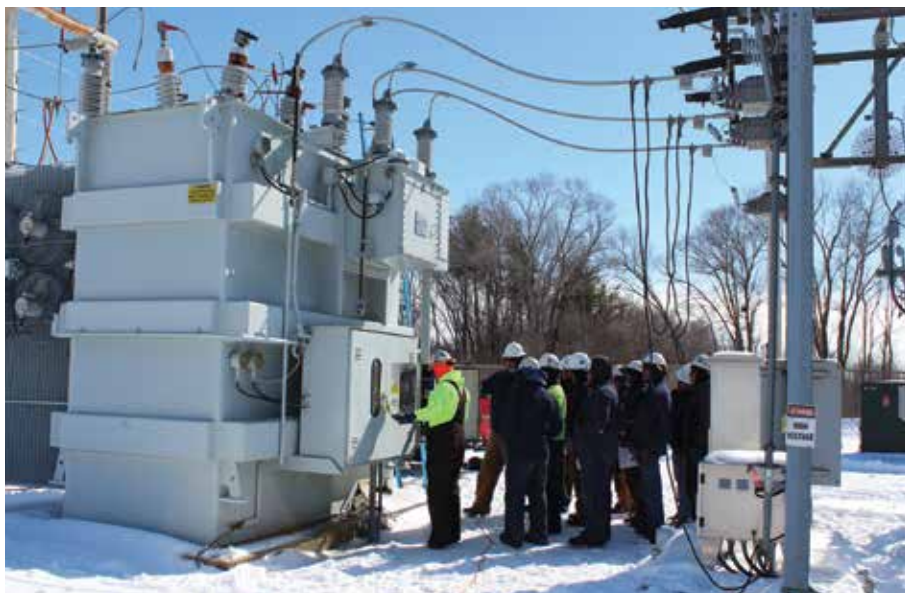
Regular maintenance keeps the electricity flowing. Here, line workers learn the steps required to re-energize the Shirland Substation.
