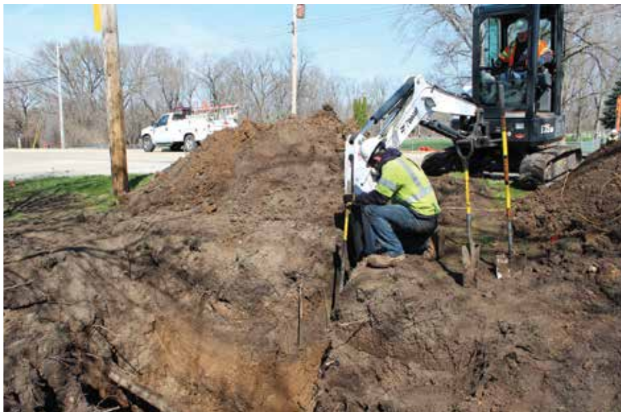
The natural gas crew replaces distribution pipe in Rockton to improve reliability and ensure safety.
